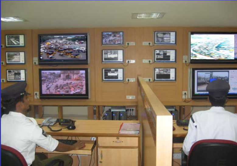
Surveillance Camera Control Room
